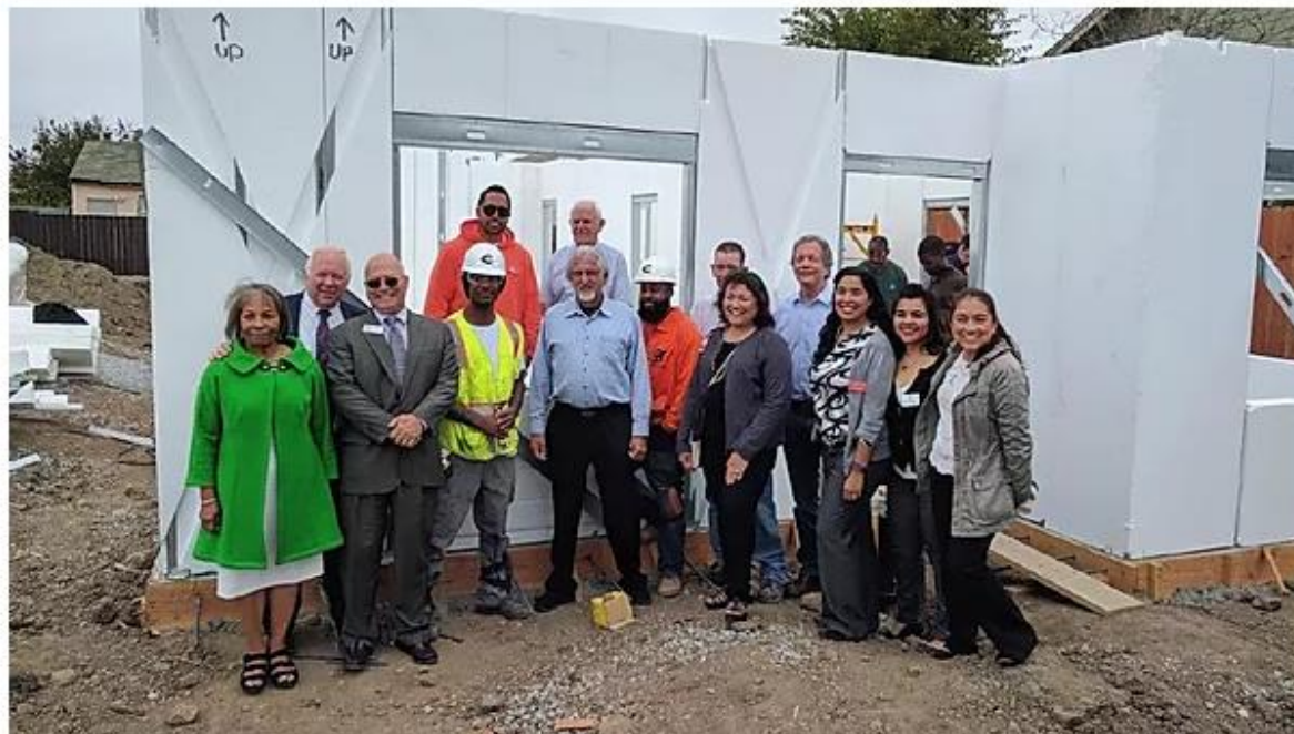
Richmond Advanced Energy Community Project Partners -- led by the Richmond Community Foundation, ZNE Alliance, the City of Richmond, Energy Solutions, and Mechanics Bank -- celebrate the construction of a Zero Net Energy Home
