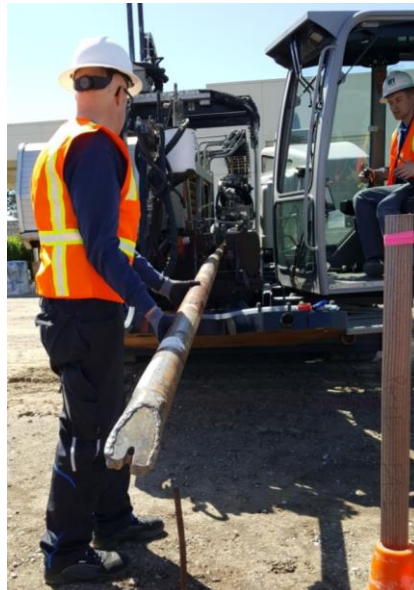
Installation of the Orfeus rod on a boring machine at PG&E in October 2017
