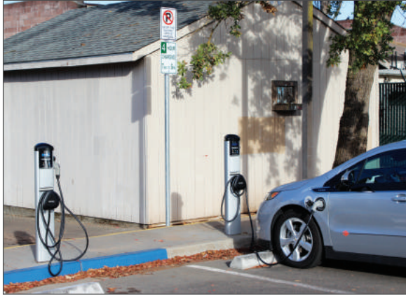
ChargePoint charging stations in the City of Sonoma, with signage and an ADA accessible parking spot.
