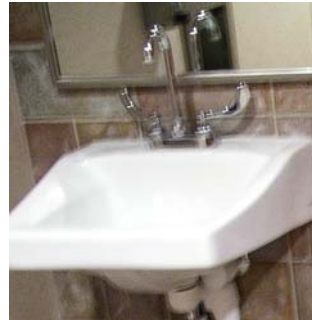
Existing Faucet – handicap stall
