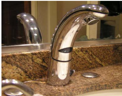
Sensor-operated Faucet – general area
