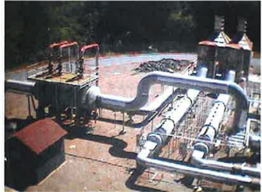
Steam Separator and Stacking System
