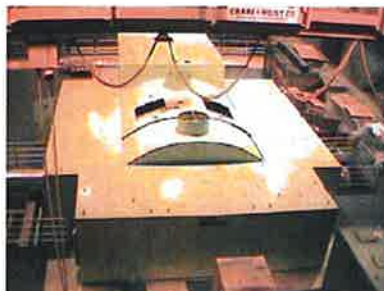
Turbine Generator (top)
