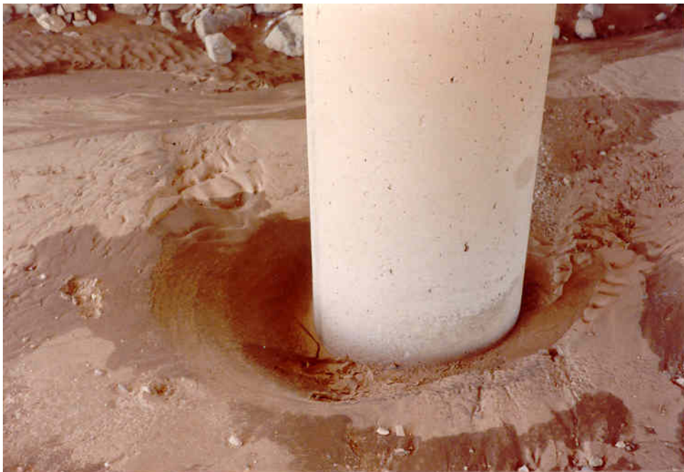
Figure 1. Local scour around bridge pier
