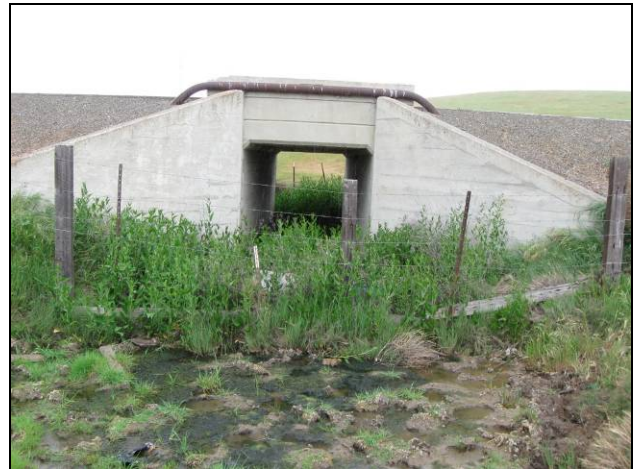
DRAINAGE WETLAND (D-1) Looking west; 6-foot by 6-foot box culvert under Bruns Road
