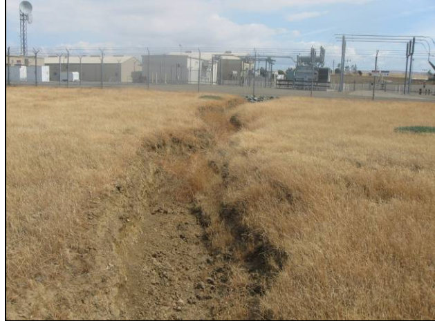
E-2 Erosional feature; looking south toward the PG&E Kelso Substation
