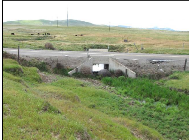
DRAINAGE WETLAND (D-3) Looking west; 6-foot by 6-foot box culvert under Bruns Road
