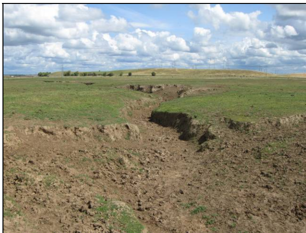
DRAINAGE (1B) North of Kelso Road, looking northeast at defined earthen channel
