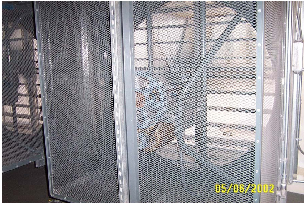
Figure 104. Relief Fan (one of six per penthouse)
