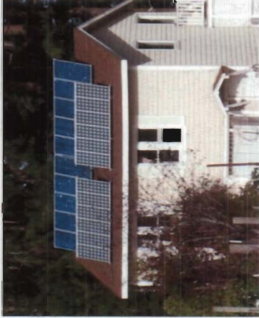
Modules installed on racks
