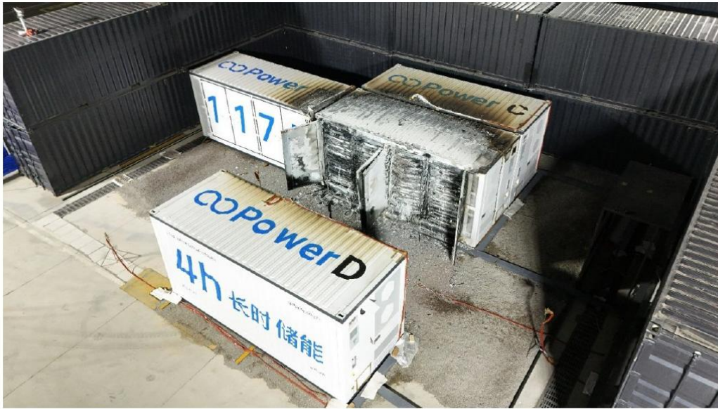
Figure 54 – Top view of post test
