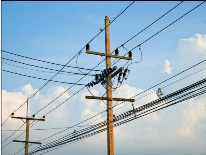
Typical distribution line ( <50 kilovolts [kV])
