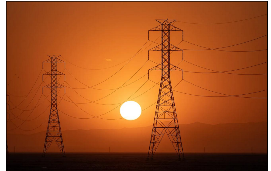
Typical transmission line ( >200 kV)
