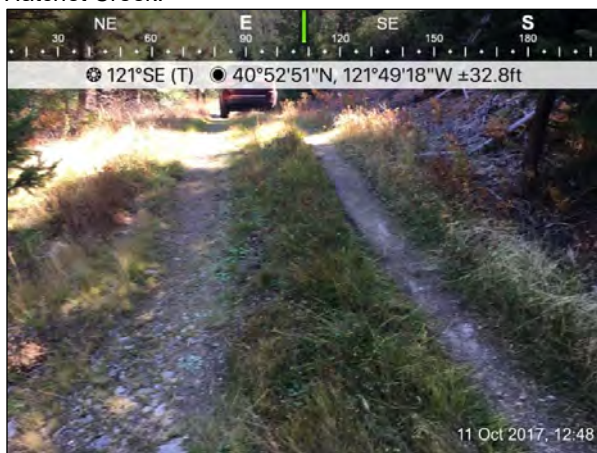
Photo 4. Wetland seep spring along an access road.
