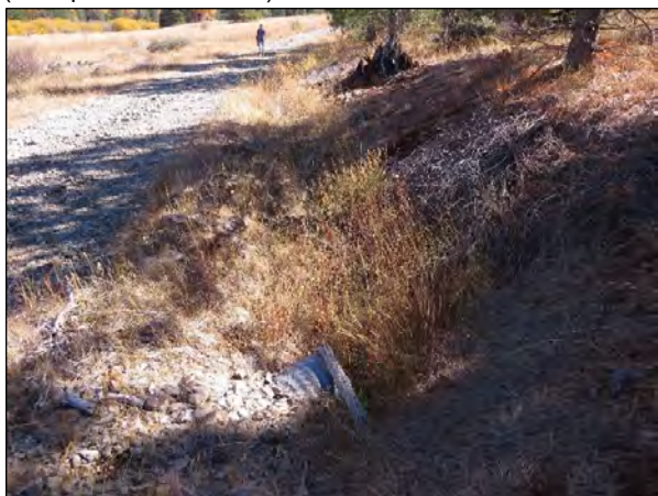
Photo 9. Non-vegetated ditch (data point 15). Orientation: northwest.
