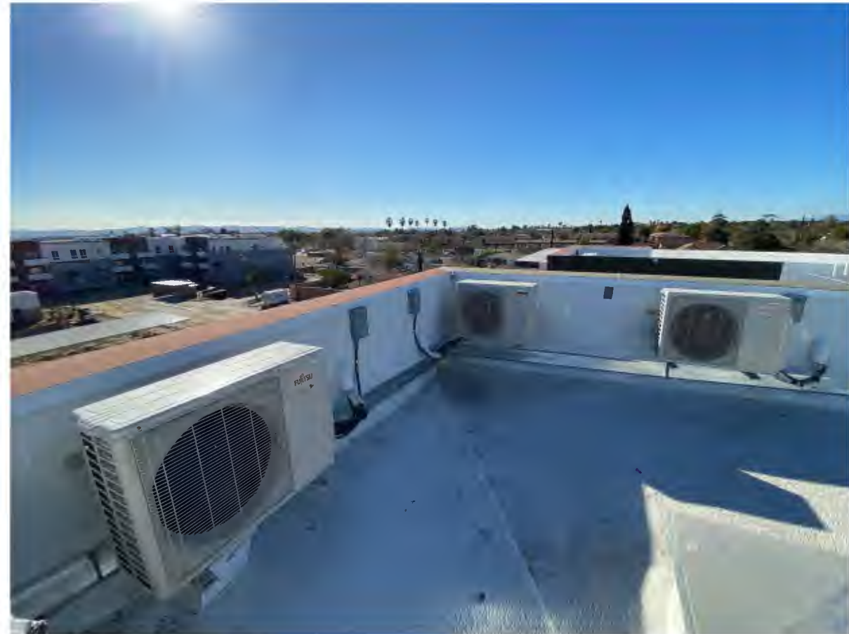
Ducted Minisplits – parapet mounted Condensers
