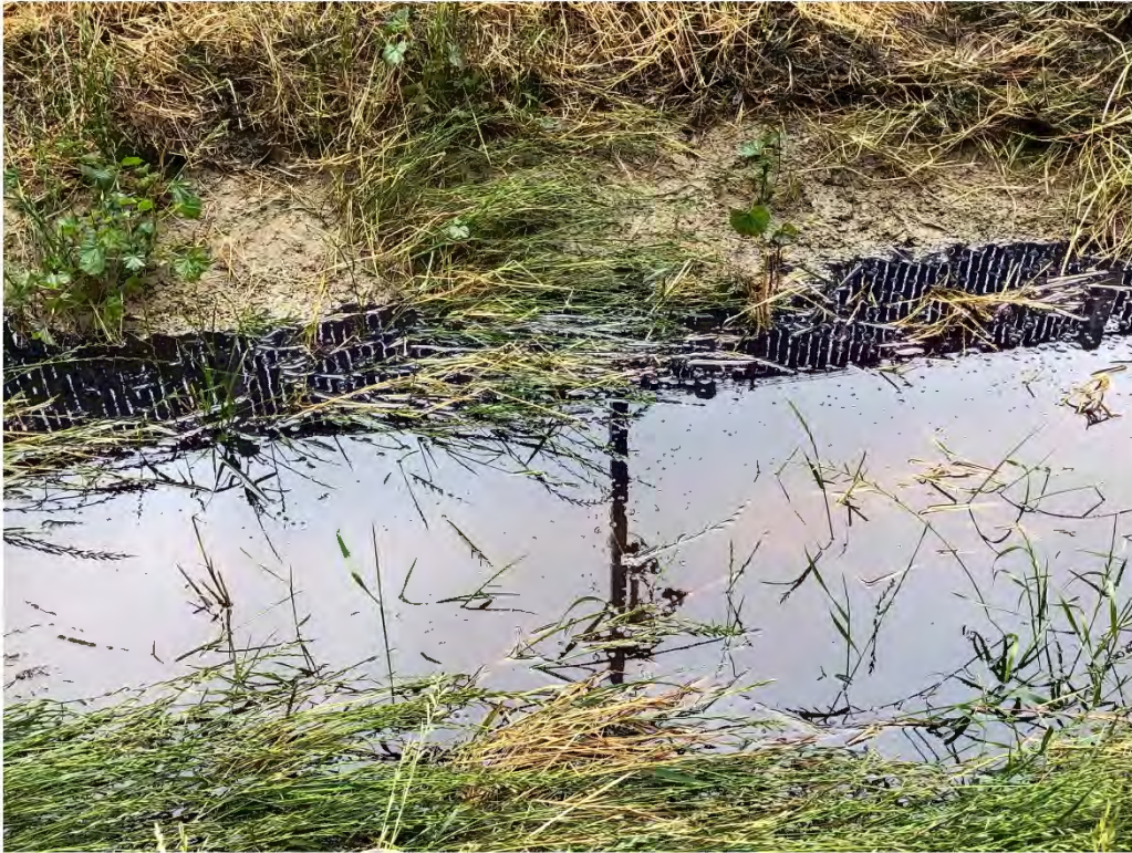
Photo 11. Close-up view of stormwater collection channel.
