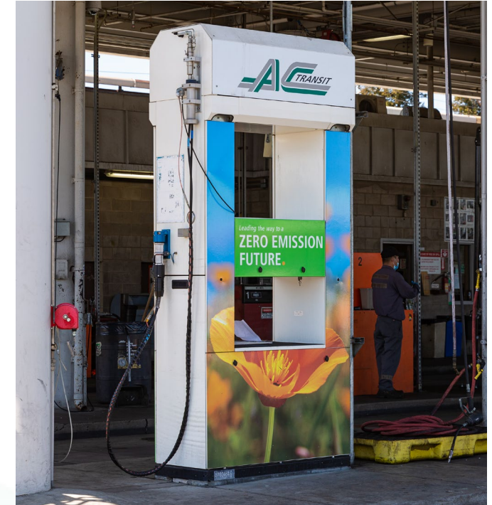
Charging and hydrogen fueling for MDHD ZEVs
