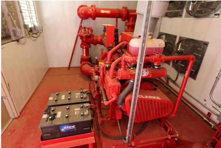
S-6 Emergency Fire Pump
