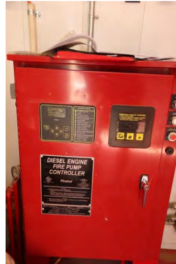
S-6 Control Unit
