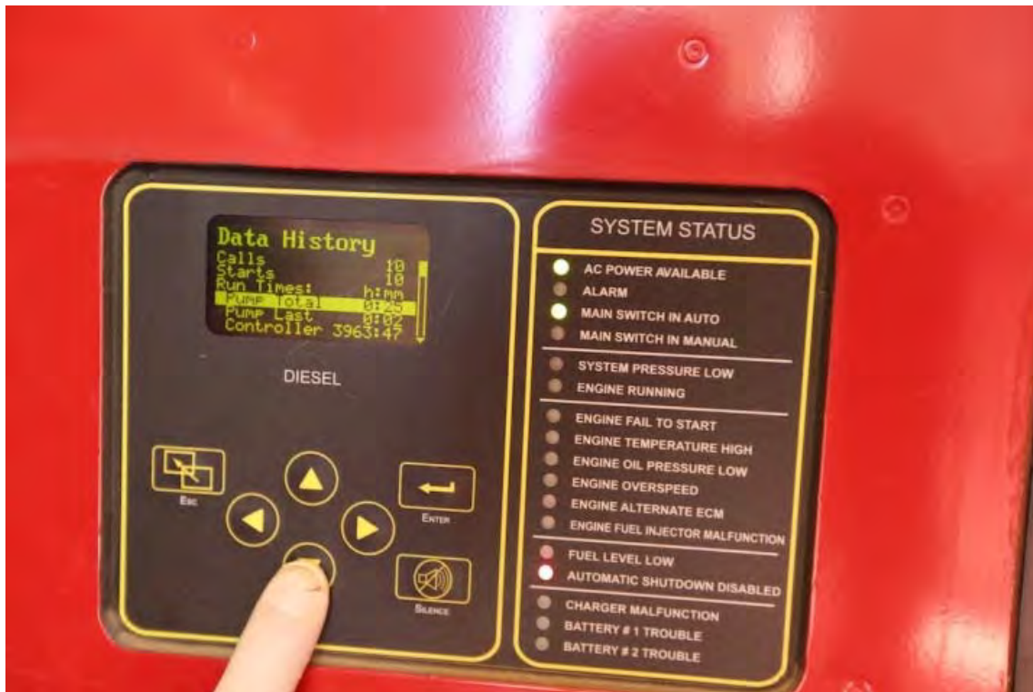
S-6 Controller, Showing Fire Pump Operating Hours
