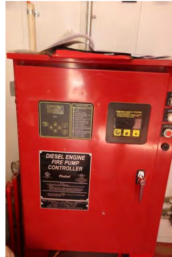
S-6 Control Unit
