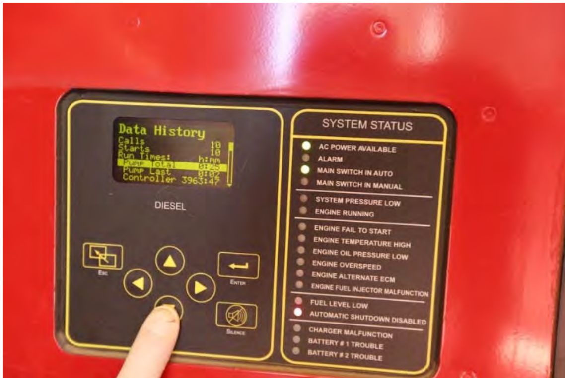
S-6 Controller, Showing Fire Pump Operating Hours
