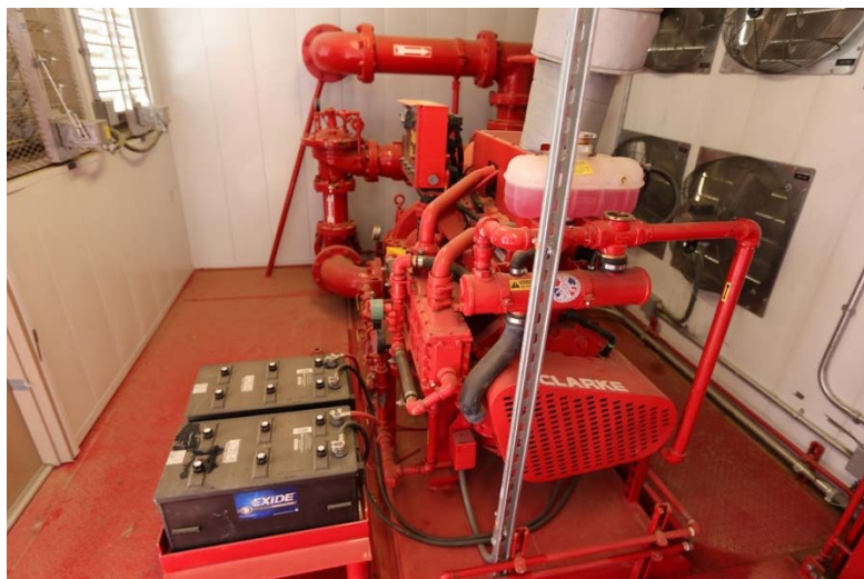
S-6 Emergency Fire Pump
