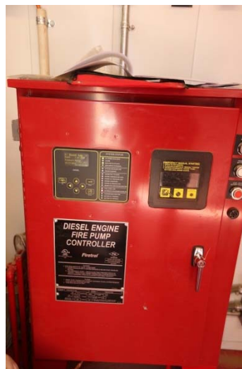
S-6 Control Unit
