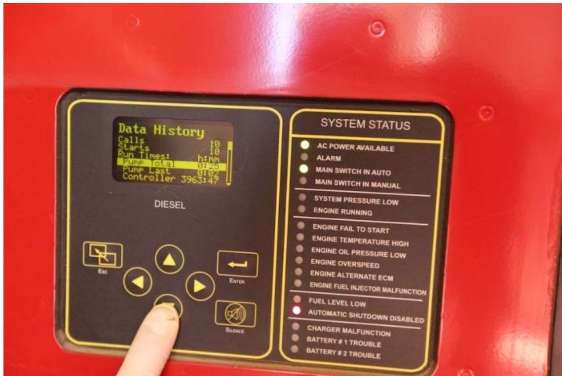
S-6 Controller, Showing Fire Pump Operating Hours
