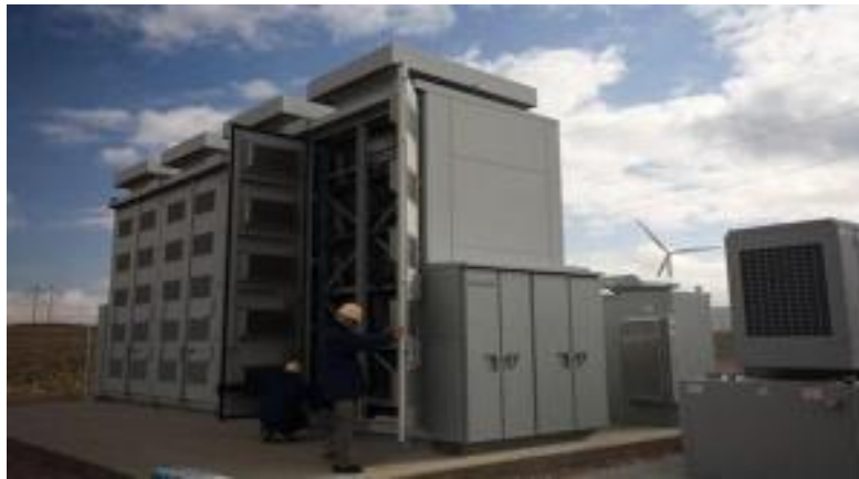
Figure 3 Lead-Acid Battery Storage
