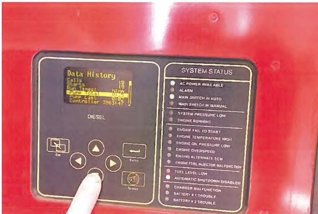
S-6 Controller, Showing Fire Pump Operating Hours
