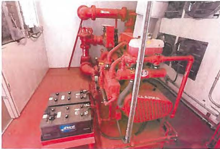
S-6 Emergency Fire Pump
