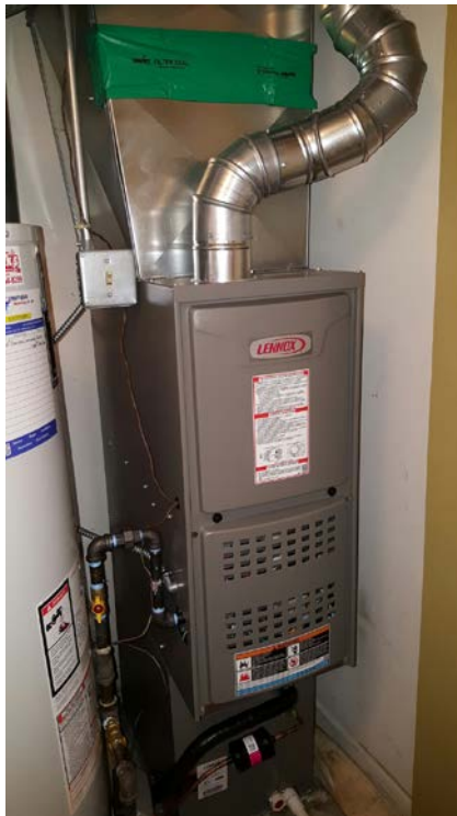
Space heating: the gas version
