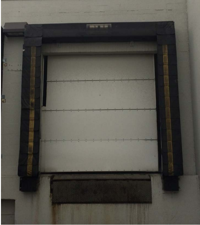
Figure 1: Loading dock with seal
