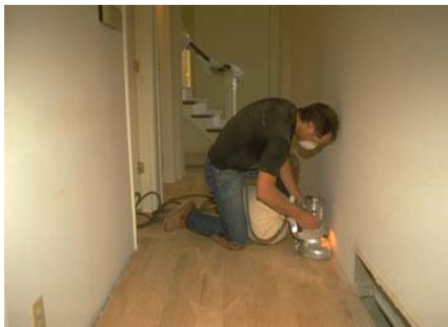
Workers who work in some non-industrial workplaces can experience harmful exposures to indoor air pollutants.
