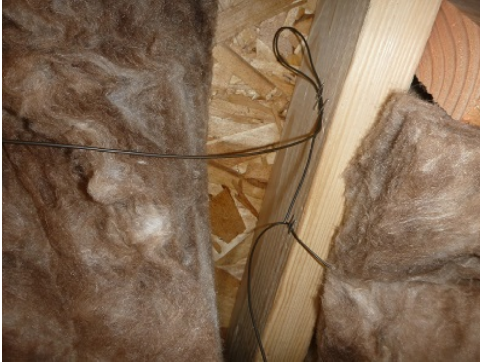
Figure 3: Example batt cabling securement method (note: insulation moved for photo).
