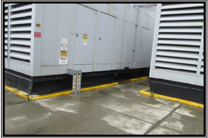
PHOTO 2: Typical self-sheltered backup generator units.
