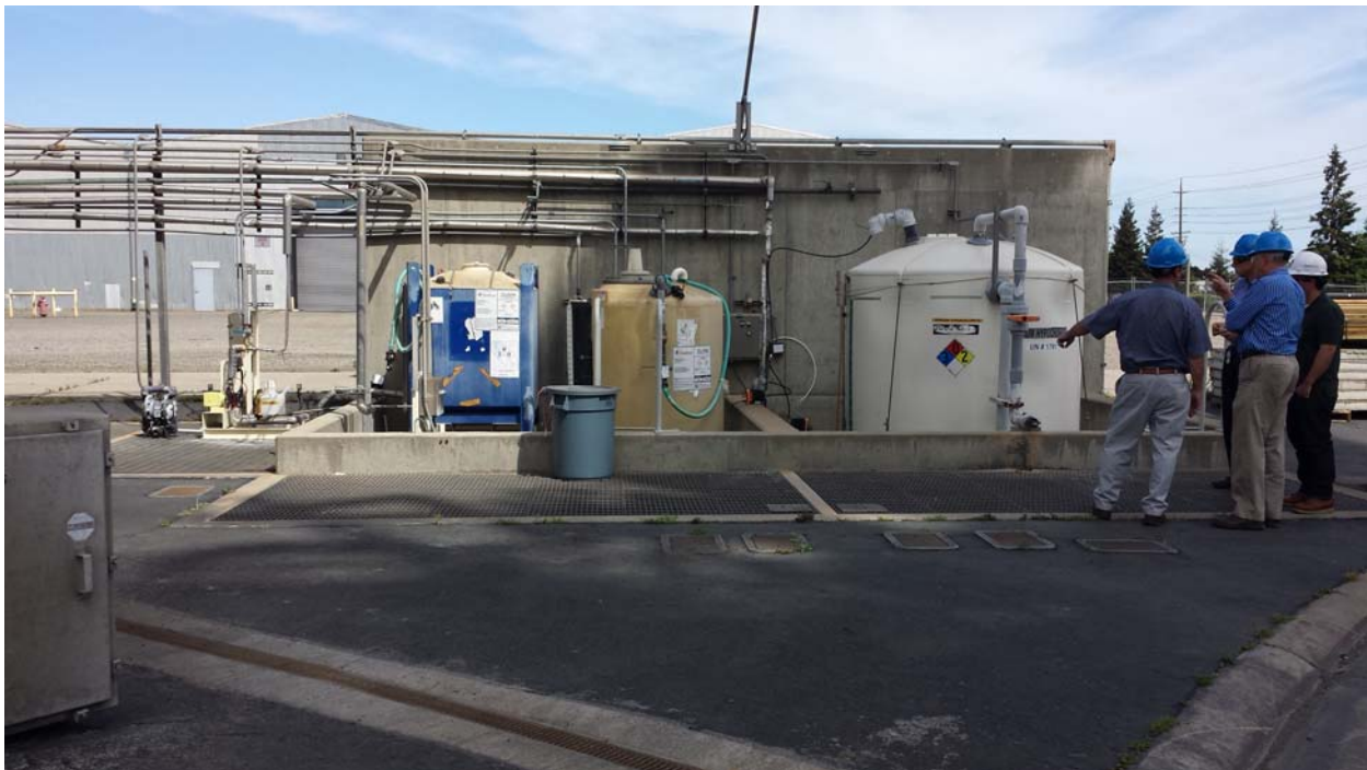
Photo 4. Sodium hypochlorite storage tank (large tank on the right). SPA plans to replace this 2,000-gallon tank with a 3,000-gallon tank, and possibly add another 3,000-gallon tank.
