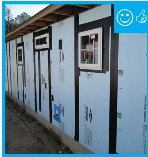
Figure 3-47 – Properly Installed Rigid Insulation with Flashing Source: 2015 International Residential Code U.S. Environmental Protection Agency
