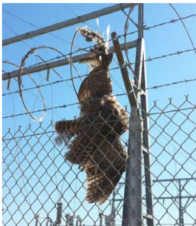
Photo 1. A great-horned owl died after becoming entangled on the razor wire placed on top of this cyclone fence. Photo by Joanne Mount.
