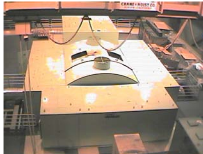
Turbine Generator (top)
