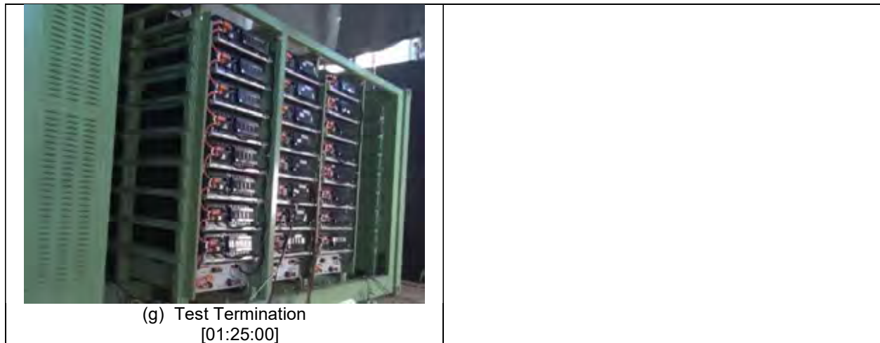
Figure 20: BESS Unit Testing Photos
