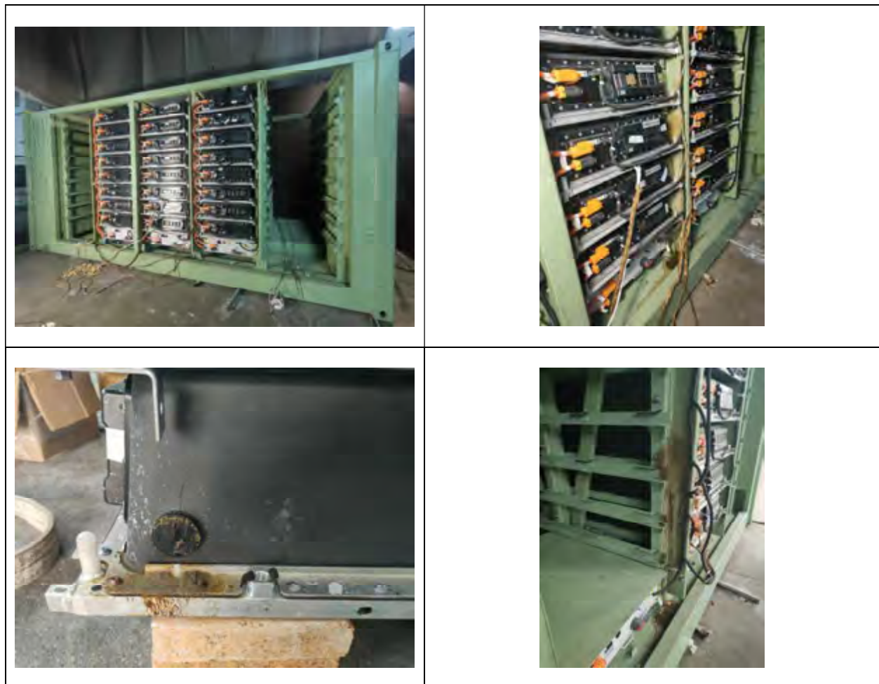
Figure 21: BESS Unit Photos after test
