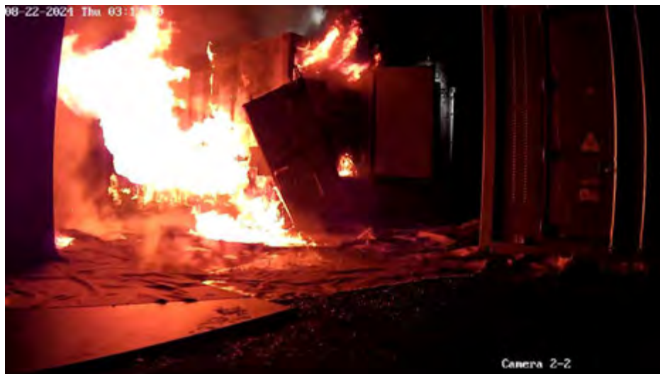
Figure 5-10 Impingement of flame jet on doors of unit C
