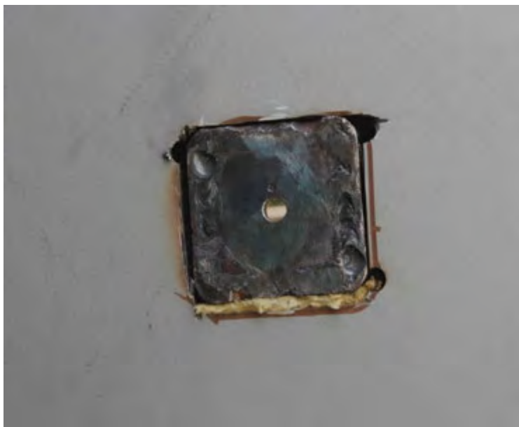
Figure 4-14 Pressure transducer well interior
