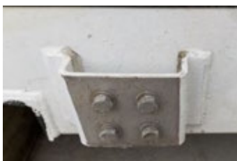
Figure 5-11 Grounding connection point
