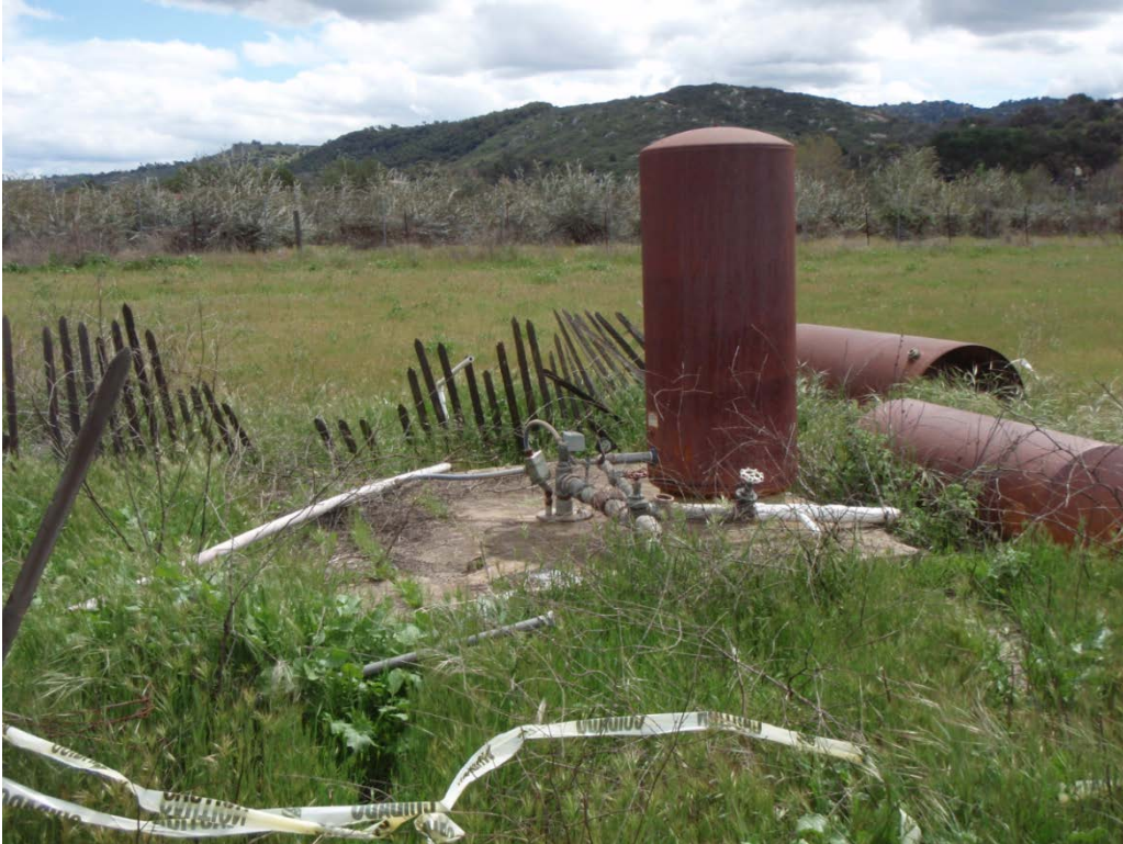
Well Head and Water Tank
