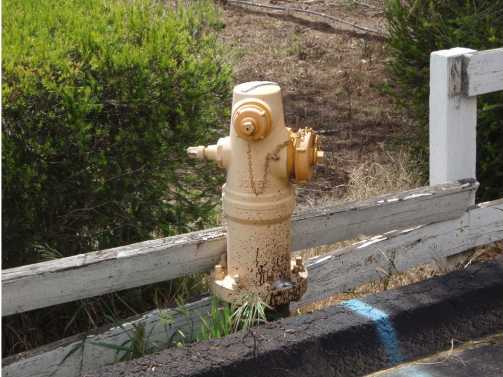
Hydrant Located at NE Corner of East Side Neighbor – Valley Center Road
