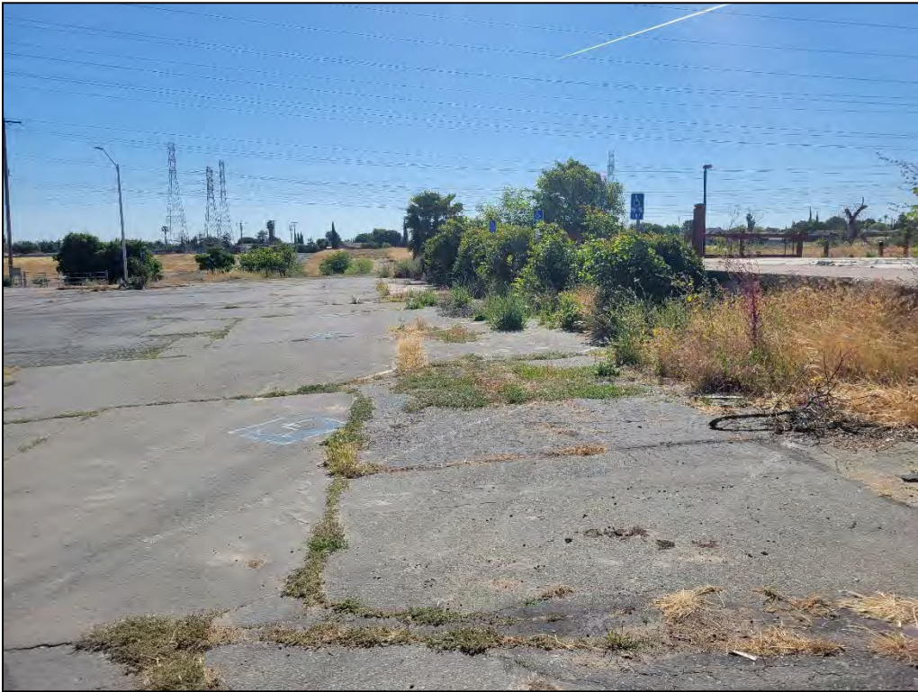
Photo 4. Representative view of the paved areas with weedy species growing in asphalt cracks. (5/19/2023)
