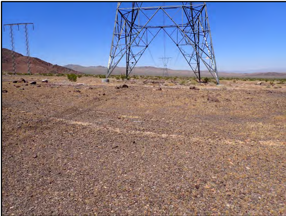
Photograph 6. Electrical transmission line going through the substation portion of the subject property northwest of I-15.
