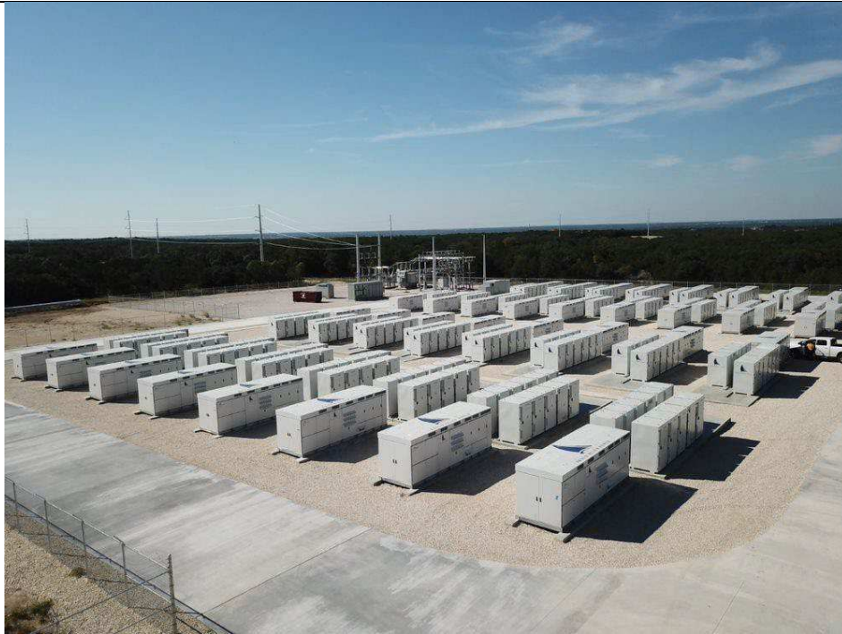
Photo 1 – Broad Reach Power LLC’s fully operational North Fork Battery Project in Williamson County, Texas.
