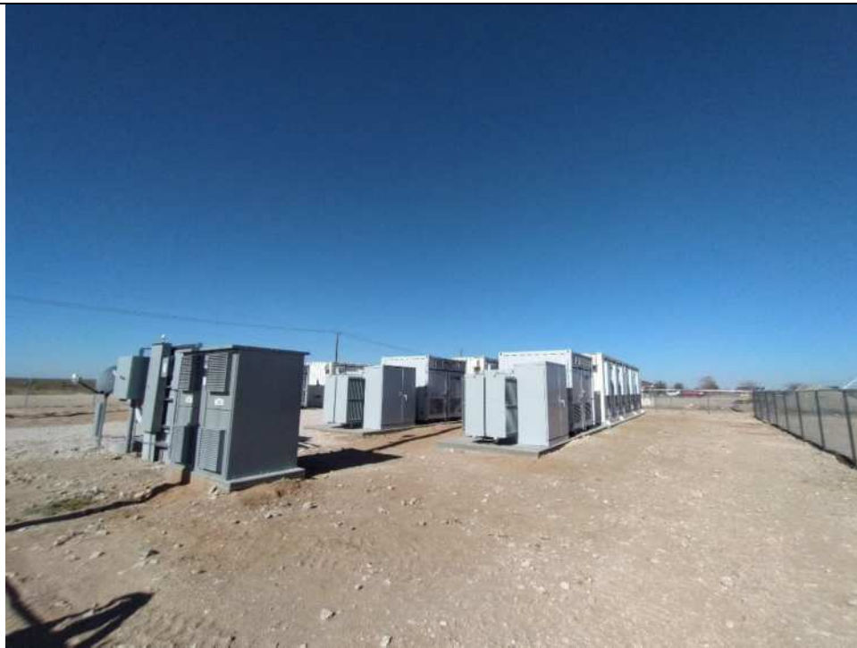
Photo 3 – BESS facilities and SCADA located within a fenced perimeter.
