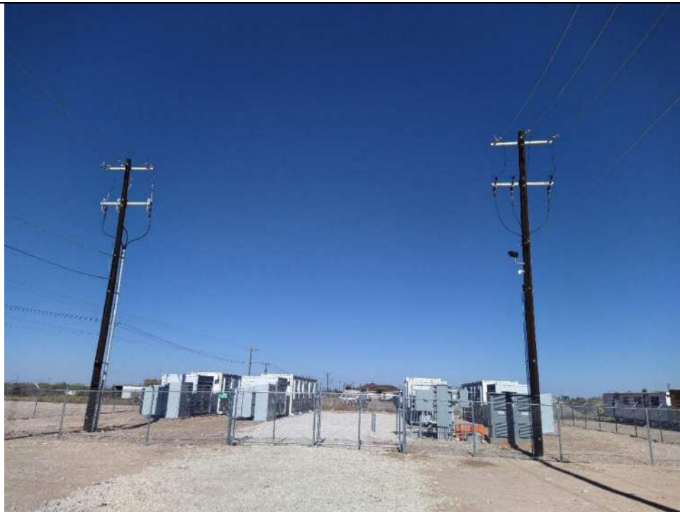
Photo 2 – Overview of the BESS facilities located within an enclosed chainlink fence.
