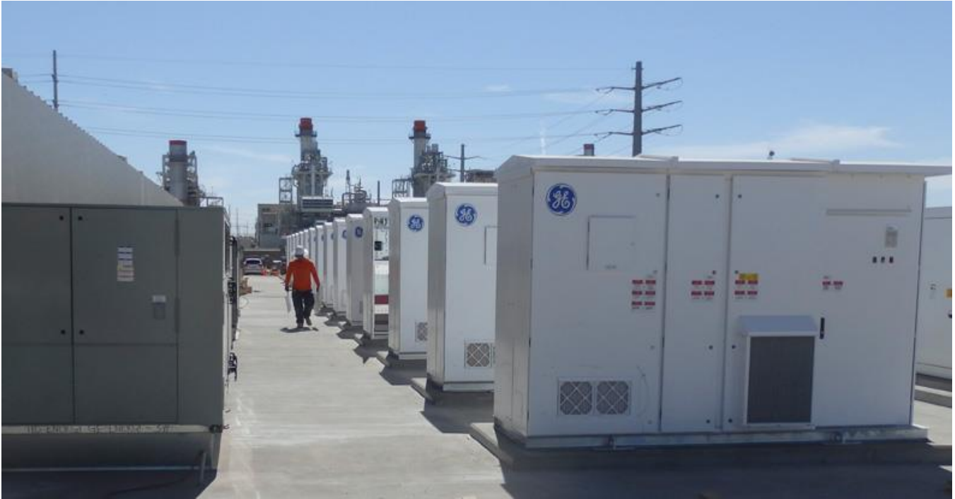
The District's 30MW Battery Energy Storage System (BESS) next to El Centro Generating Station
