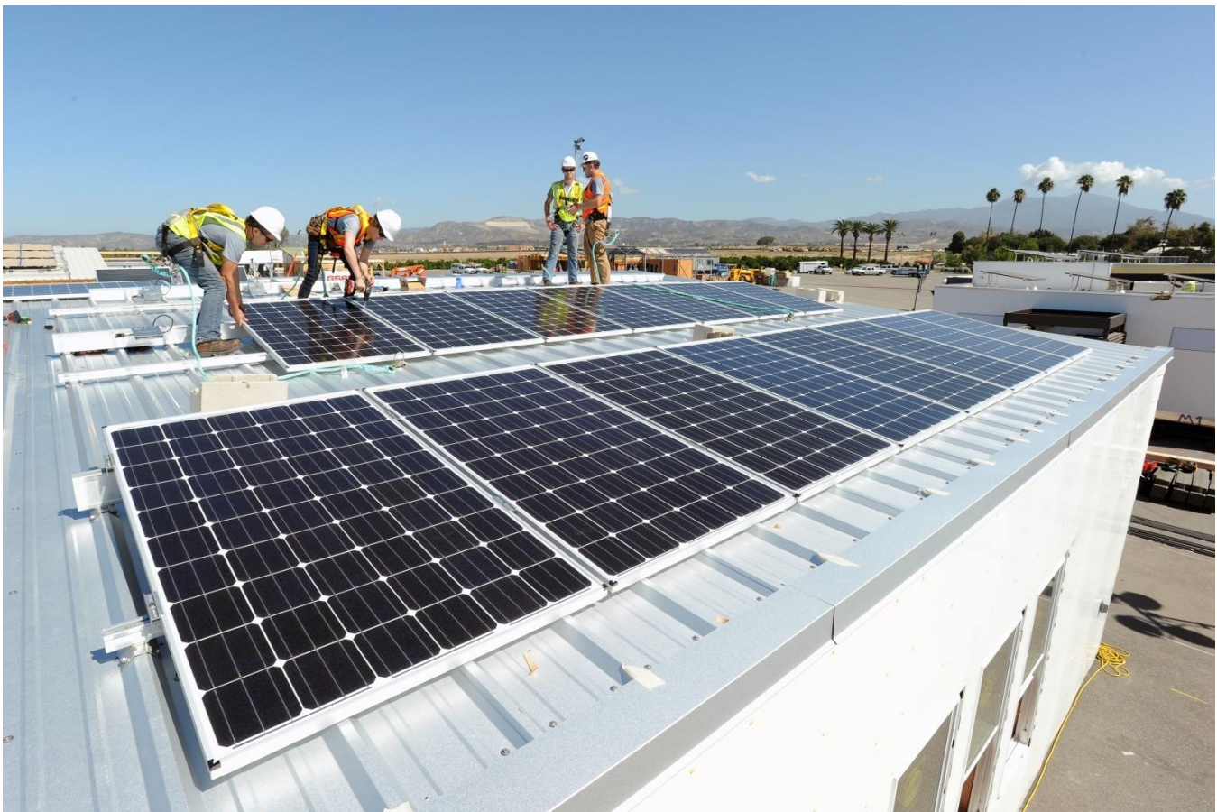
Rooftop solar installation in California. Credit: Thomas Kelsey/U.S. Department of Energy Solar Decathlon
