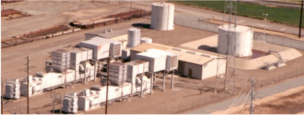
Figure 11. Walnut Power Plant
