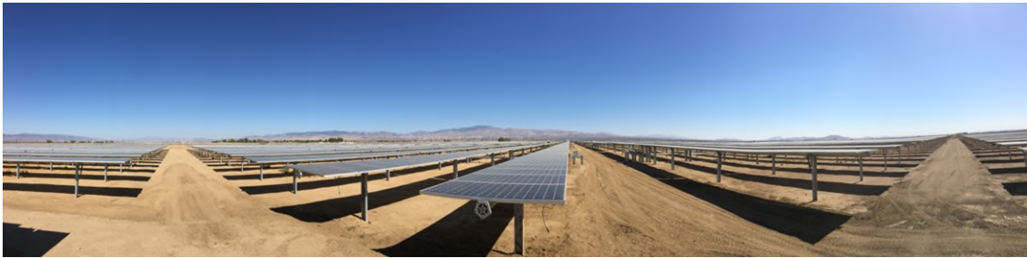
Figure 15. Rosamond West Solar 2 Facility
