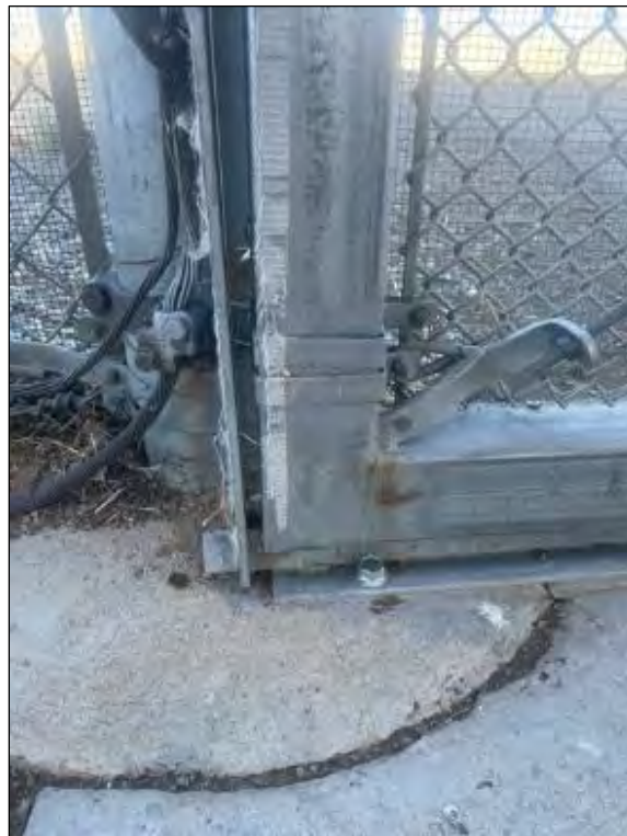
Photo 17. One and a half inches of clearance between the bottom of the gate and the road, a potential entry point for rattlesnakes found on June 1 st , 2022.
