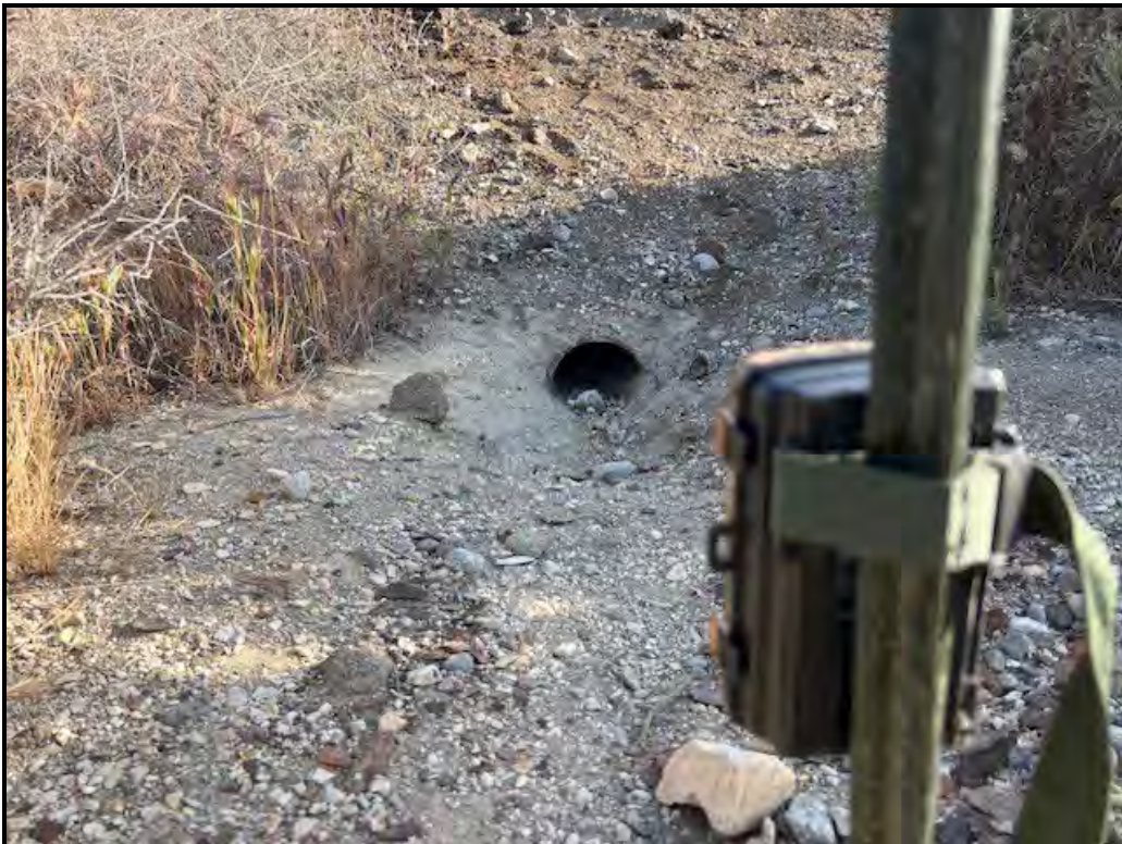
CT10 (35.21190, -119.58513): Located well beyond the perimeter fencing at an open culvert in the northern northwestern portion of the Site
