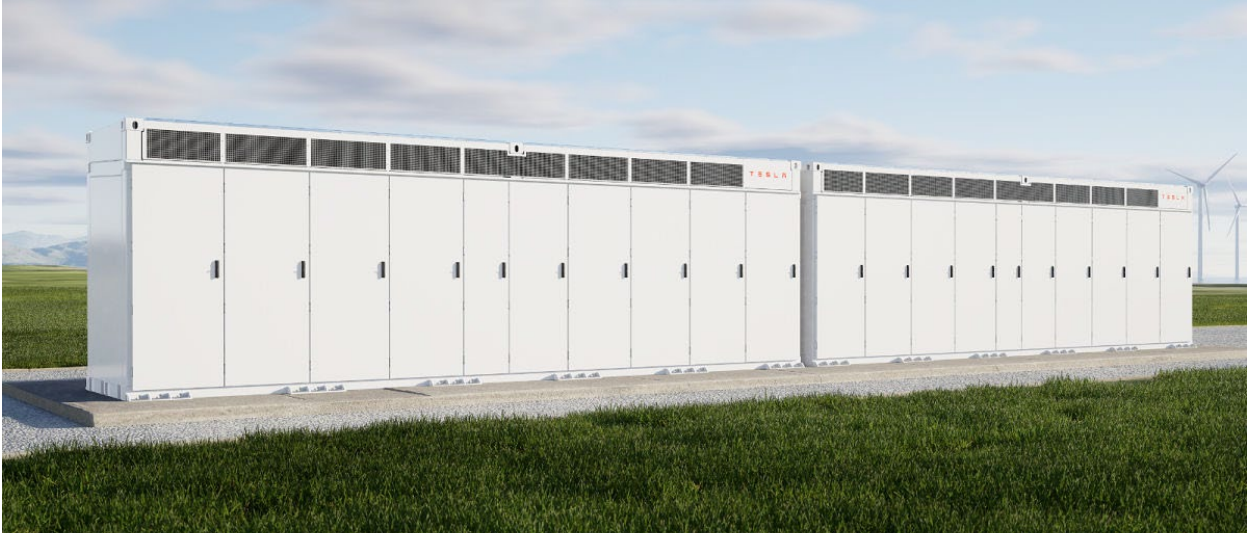
Figure 2.3-6 Battery Energy Storage System Example Technology
