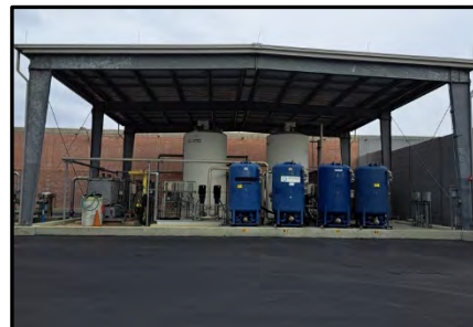
RO Skid Structure (1/24/24)
