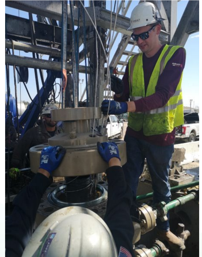
Installation of distributed fiber optic sensing in a gas storage well Source: LBNL
