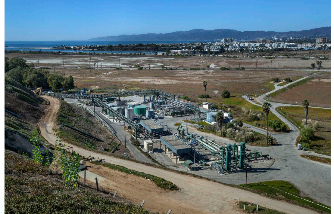
SoCalGas Playa del Rey underground gas storage facility Source: LA Times
