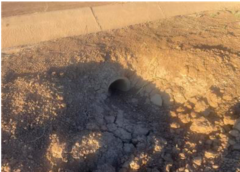
Photograph 3: BUOW_06 - Culvert being used as a burrow in BRGP BSA. This culvert is not managed by the IID.
