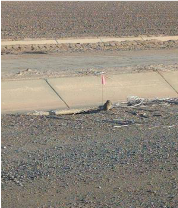
Photograph 2: BUOW_05 - Burrow in BRGP BSA under the edge of a concrete canal. This canal is managed by the IID.
