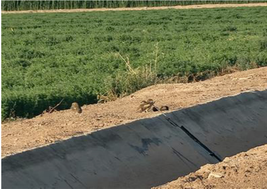
Photograph 12: BUOW_23 - Burrow in ENGP BSA under the edge of a concrete canal. This canal is not managed by the Imperial Irrigation District IID.
