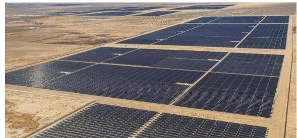
Figure 52. Astoria II Solar Photovoltaic Facility
