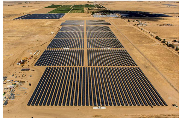
Figure 53. Antelope DSR 1 Solar PV Facility
