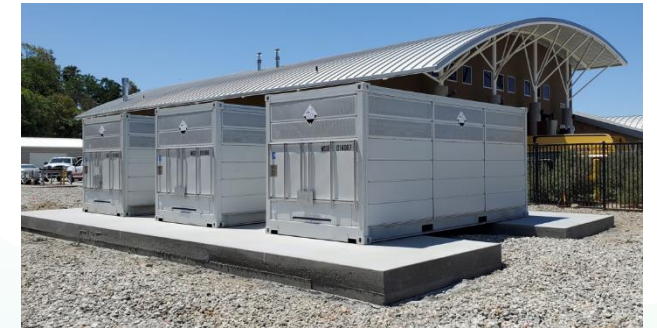
EPC-19-045, Invinity Vanadium Flow Battery installed at the fire station run by the Soboba Band of Luiseno Indians
