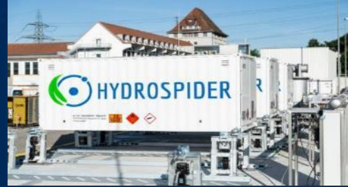
Hydrogen production & container H 2 production nearby power plant
