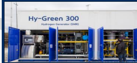
Hydrogen production plant
