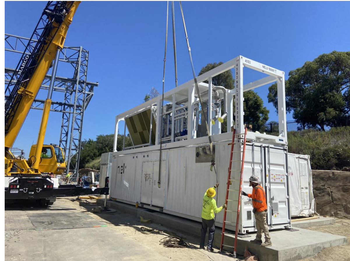
Electrolyzer Delivery, August 2023 Palomar Energy Center, Escondido, CA
