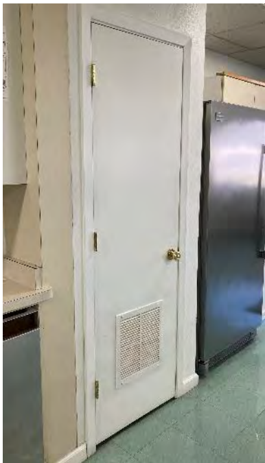
Figure 45: DHW closet door with lower grilles from a small commercial kitchen in Woodland, CA.
